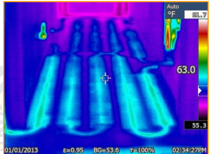
PROPERTY INSPECTOR Radiant heating installed
